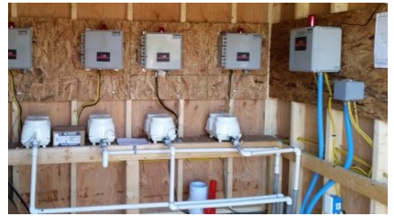
Multiple system configurations may be controlled independently (shown) or by one customized controller.
